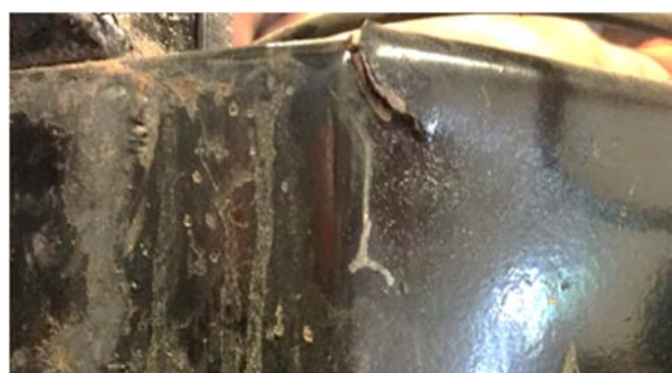
Figure 14. Cracking from sharp corners in frame
