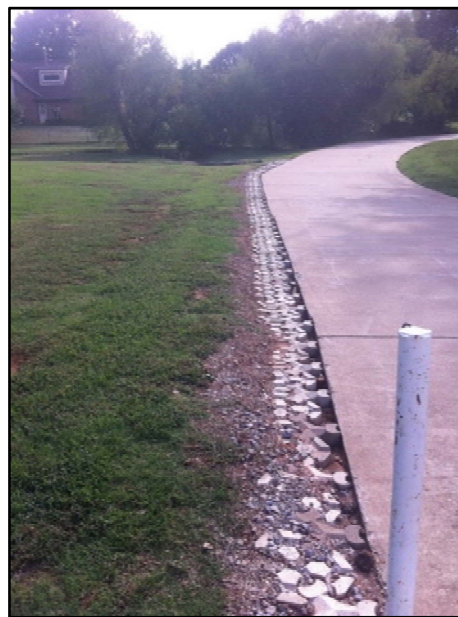
Figure 27. Soil Erosion along Pool Driveway Entrance at Site C
