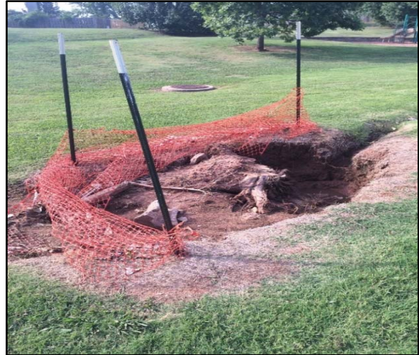
Figure 3. Example of Erosion in Greenbelt Area
