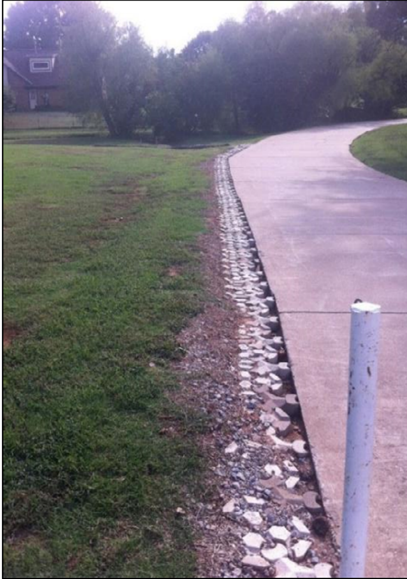
Figure 41. Soil Erosion along Pool Driveway Entrance at Site C
