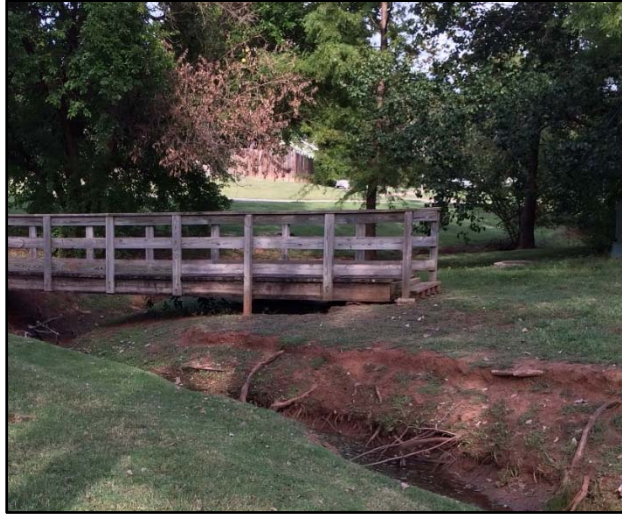
Figure 4. Erosion near Walking Bridge
