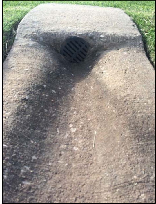
Figure 15. Undersized Drain at Park View Estates
