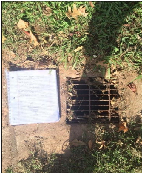
Figure 35. Undersized Storm Drain at Site A
