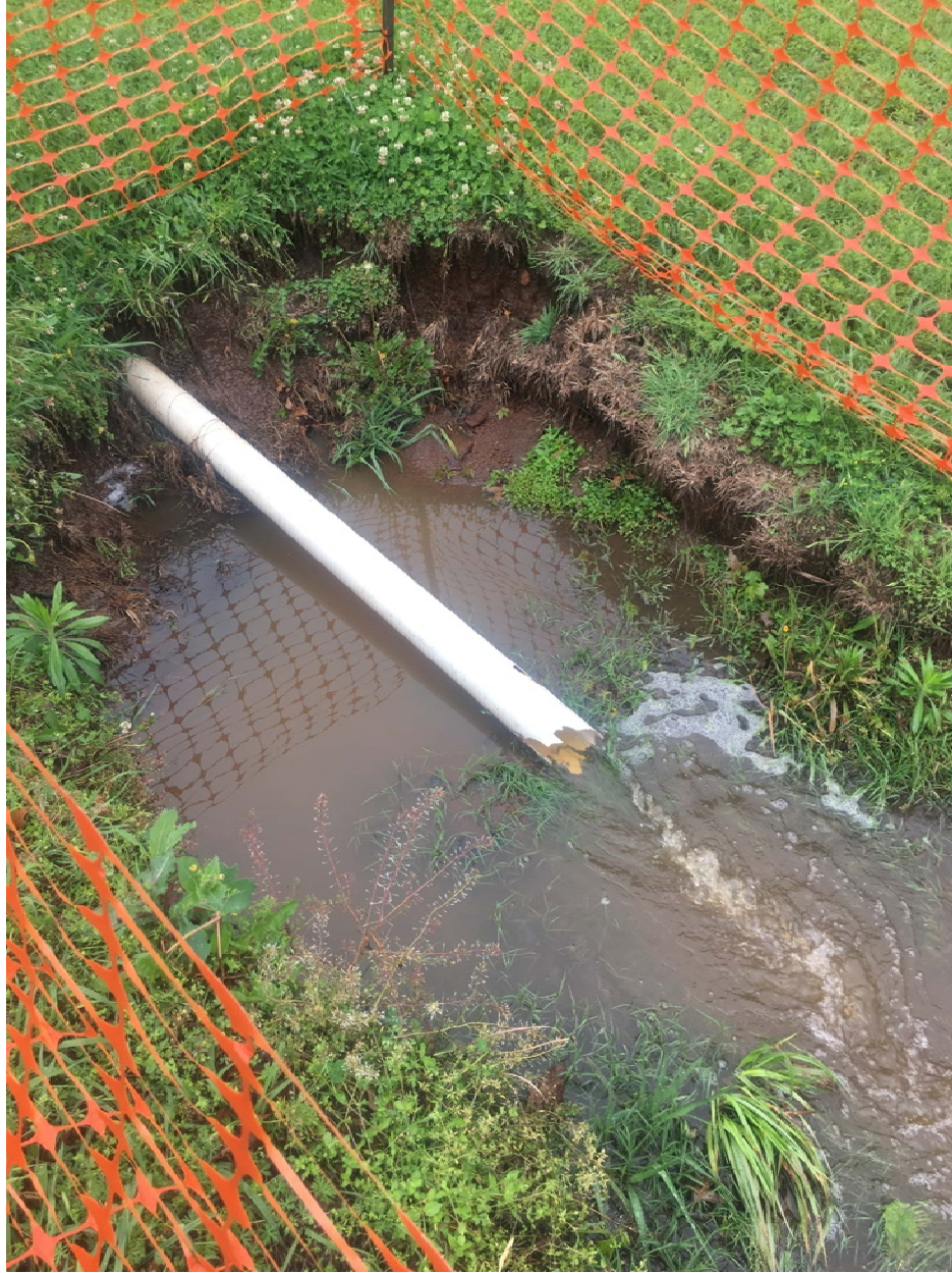
Figure 33. Erosion Caused by Broken Pipe
