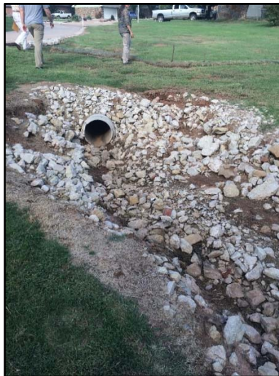
Figure 26. Erosion Occurring at Storm Culvert Outlet Located at Site C
