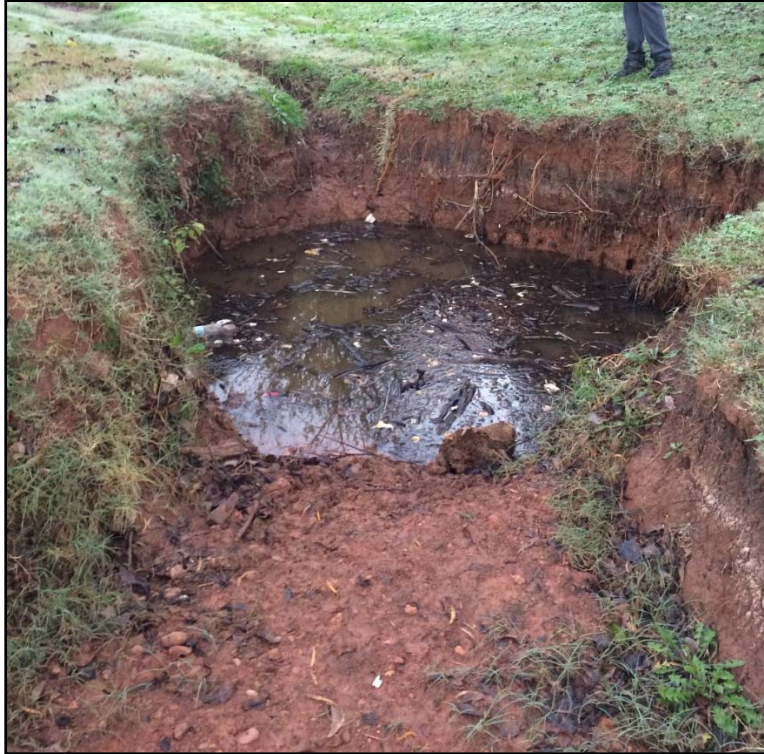
Figure 23. Example of Erosion Occurring at Site B
