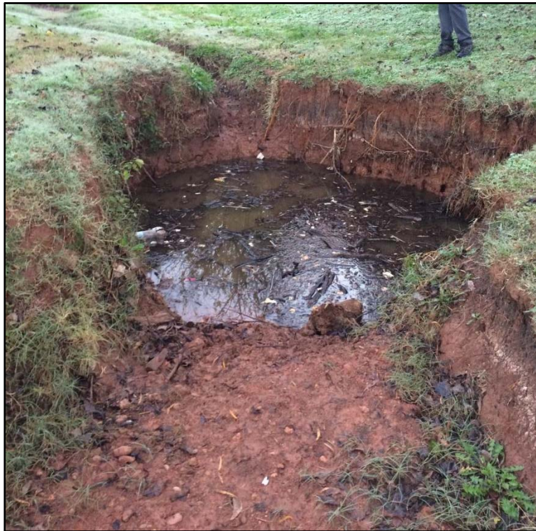
Figure 4. Erosion at Site B
