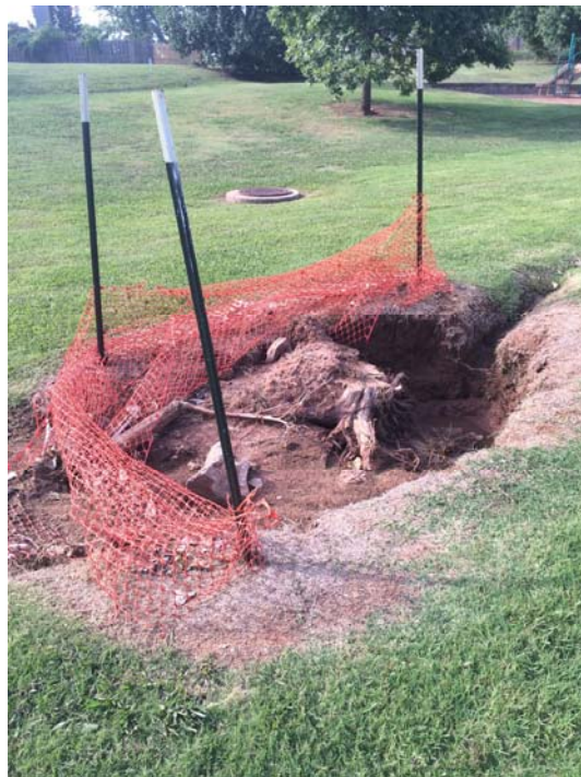
Figure 3. Erosion around Stump
