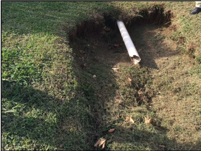
Figure 16. Erosion Caused by Pipe Blowout
