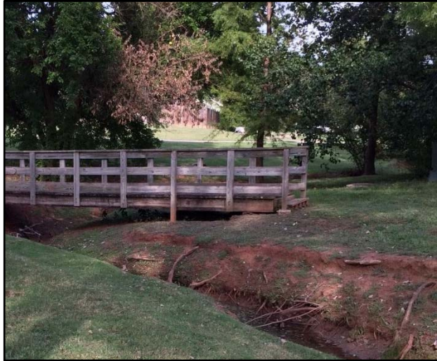
Figure 5. Erosion near Walking Bridge
