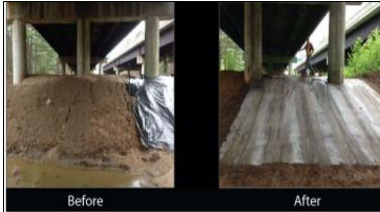
Figure 36: Example of concrete blanket effects (Milliken Infrastructure)
