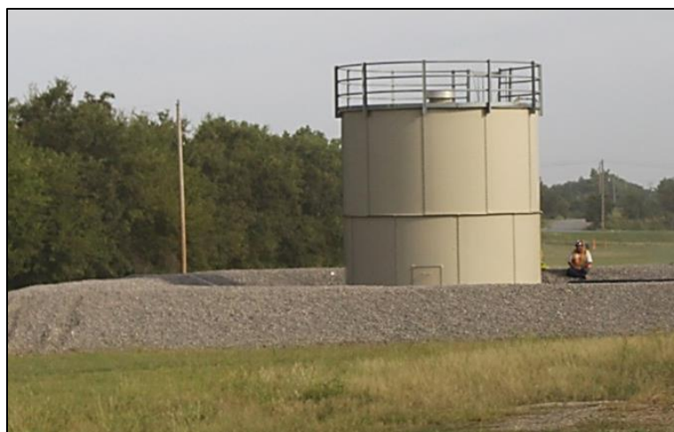
Figure 28: Enid Municipal Landfill leachate collection tank
