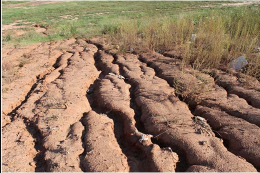
Severe Erosion Rill Formation
