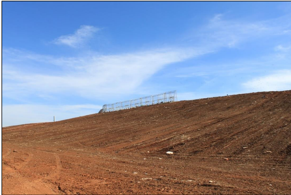
Figure 1: North-facing problem slope
