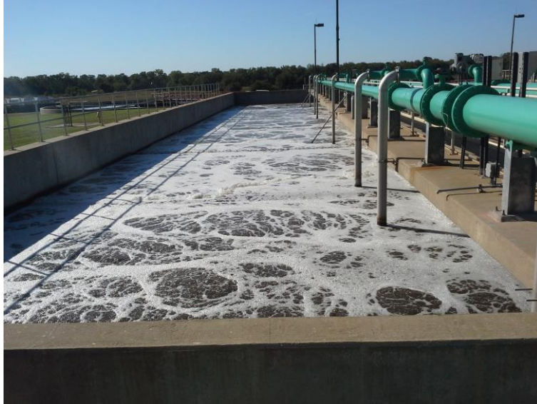
Figure 3: An aeration basin, this picture was taken at the Stillwater Wastewater Treatment Plant
