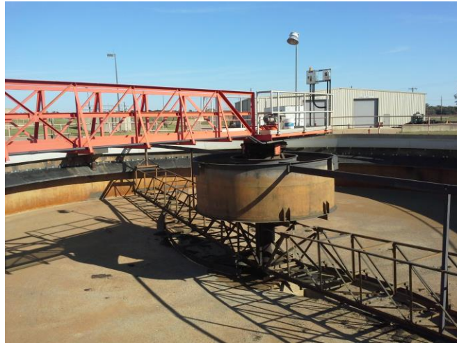
Figure 4: An empty clarifier, this picture was taken at the Stillwater Wastewater Treatment Plant.
