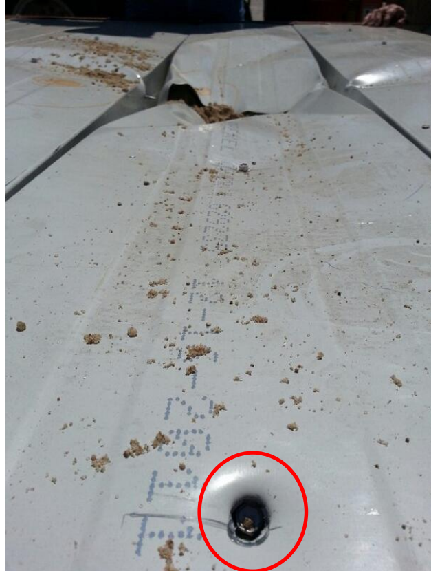
Figure 23: Screw Pull Out Resulting from Impact
