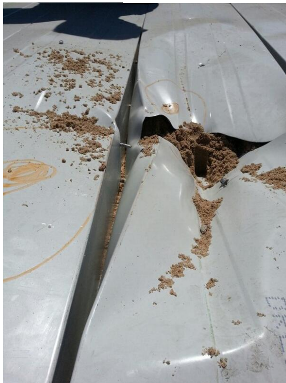
Figure 25: Puncture of Panels and Screw Pull Out Resulting from Impact
