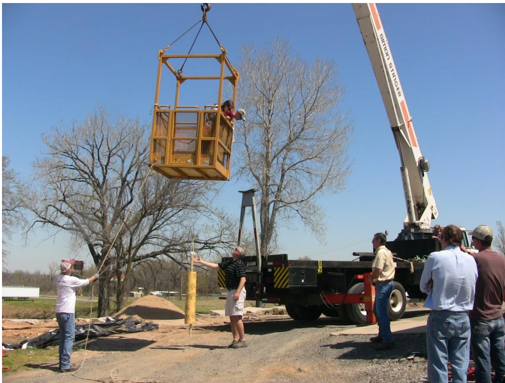
Figure 15: Making Sure Everything is Working Properly
