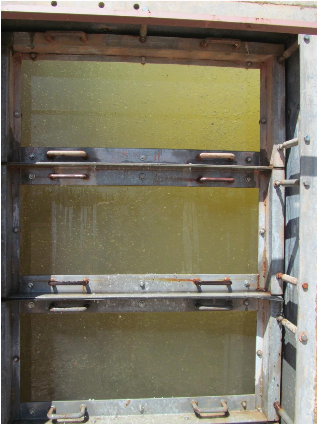
Figure 13: View through the window of mixing created by the bubble tubing.
