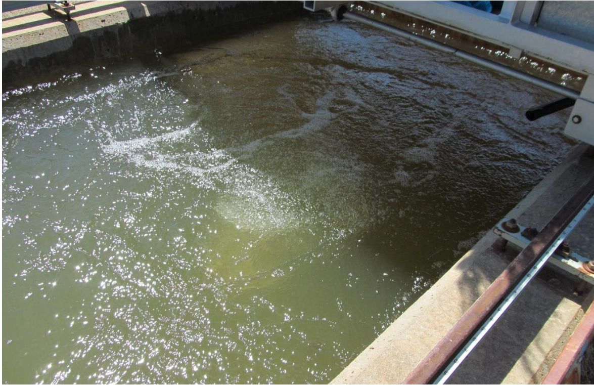
Figure 12: Diffuser #1 and #3 running at 8.5 psi, significant overlapping occurred.
