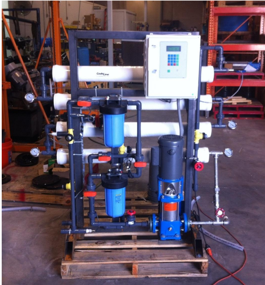
Figure 1: Pumps of Oklahoma Reverse Osmosis (RO) System
