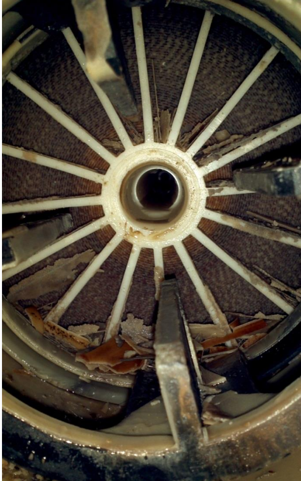
Figure 2: Iron-fouled RO Membrane (Membranes should be white)
