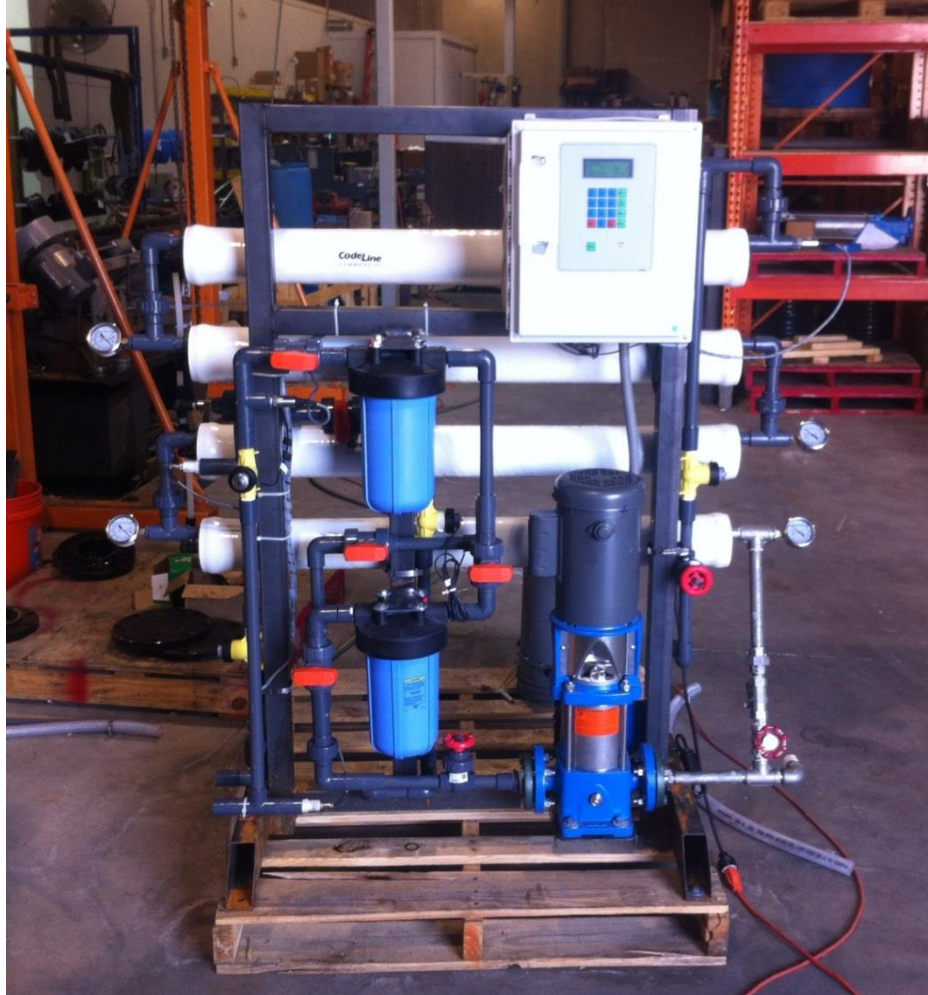
Figure 4: Pumps of Oklahoma Reverse Osmosis (RO) System
