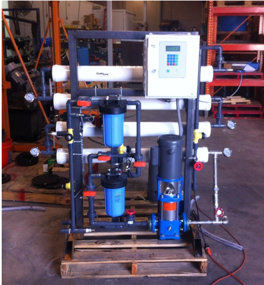
Figure 1: Pumps of Oklahoma Reverse Osmosis (RO) System
