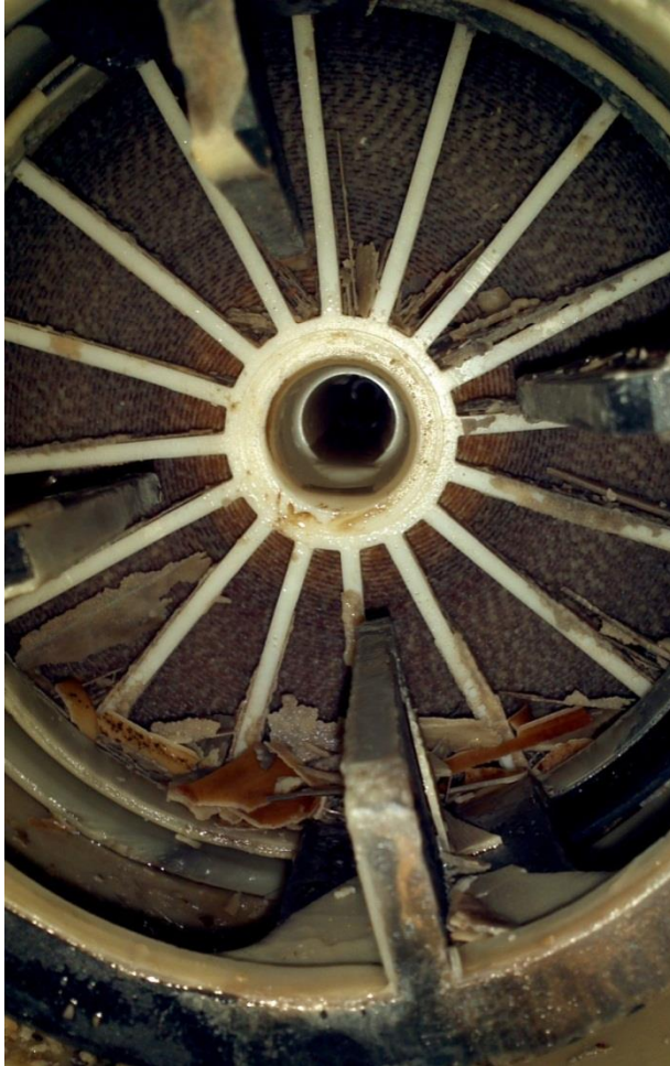
Figure 2: Iron-fouled RO Membrane (Membranes should be white)
