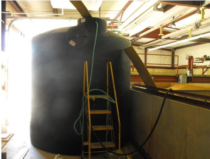
Figure 15. The Illinois River water was stored in the black tank seen above. Also shown is the small pump which took the water from the storage tank to the alum mixing tank.
