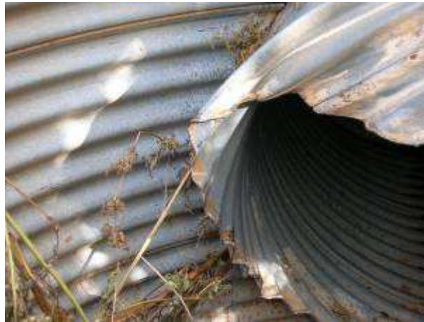
FIGURE 9 – SCHRECK'S FAILED DROP INLET STRUCTURE
