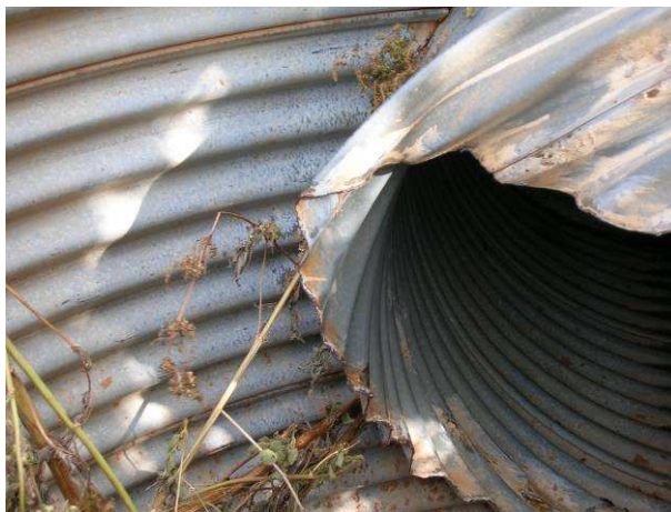
Figure 9. – Schreck's failed drop inlet structure
