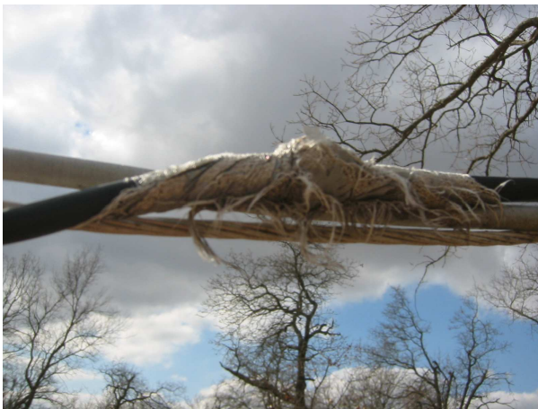
Figure 3: Damaged conductor insulation covered with tape.
