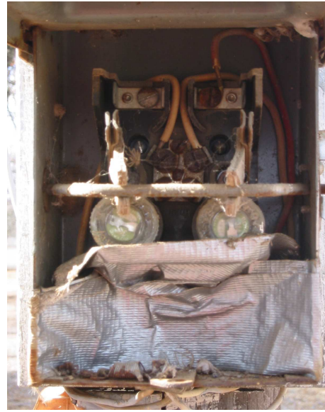
Figure 2: Damaged fuse box in disrepair
