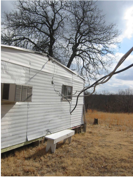
Figure 1: Low hanging electrical wire improperly attached/entering a building
