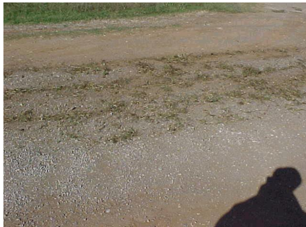
Figure 14: Lack of Consistency in Sprig Application
